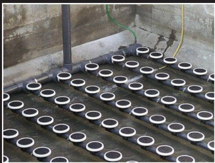
Figure 1 - Diffusion Gas Sparging array.
